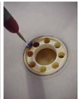
Figure17 The cause is damage to the weld between the collecting cup and sheet
